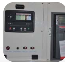
Control Panel & MCB
